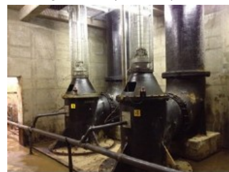
Fig 2. Original pumps from Allen Gwynnes
